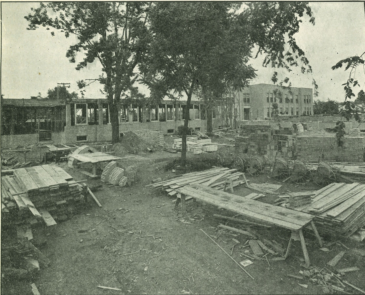
Construction is proceeding rapidly on the Administration Building and the Clara Elizabeth Knudsen Chapel
