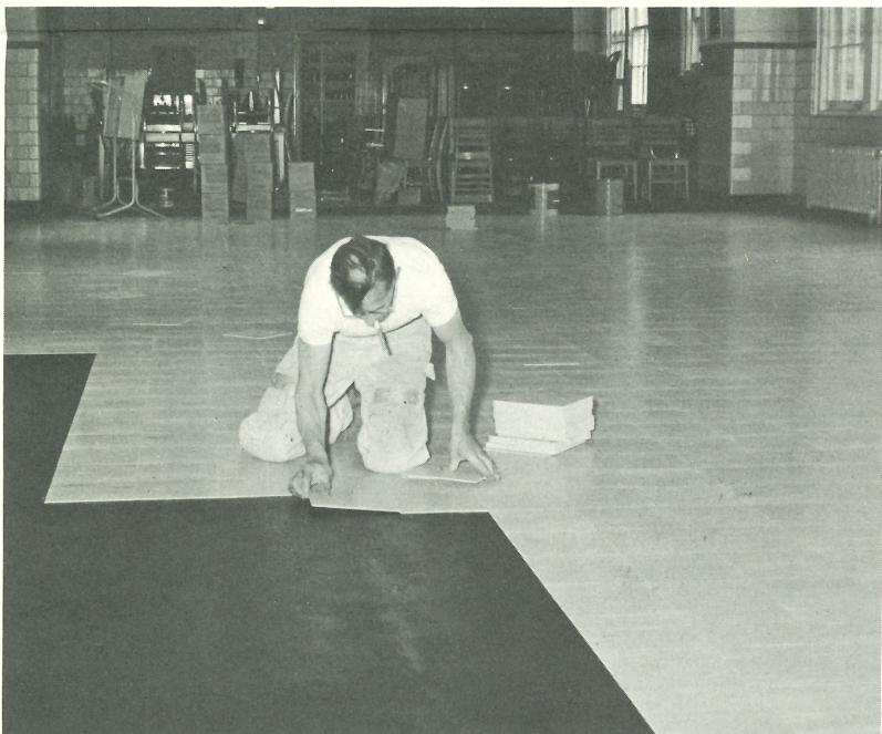
Workmen complete the laying of new tile in the school's dining room.
