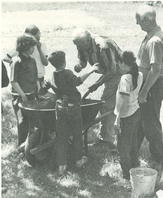
During the erection of some of the new playground equipment the children had opportunity to become acquainted with the volunteers. While mixing some cement, Mr. Schorling and Mr. Koester discuss the matter with pupils.
