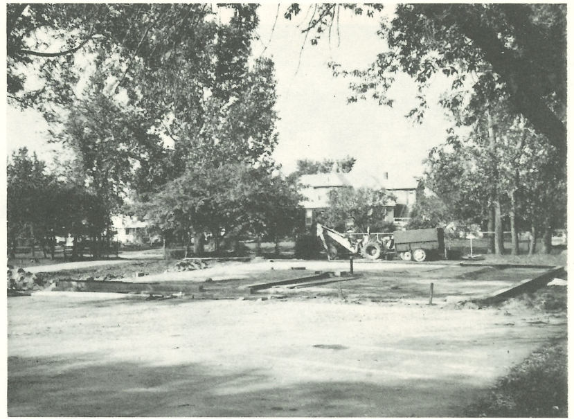
Waiting for the walls to go up. The Kresge Foundation gift makes possible the construction of a much needed garage and storage building.
